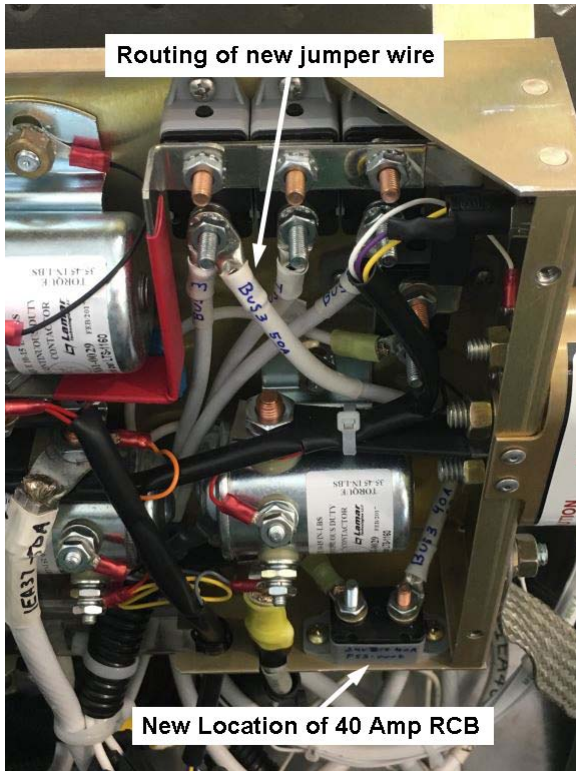
FIGURE 4 – New Location for 40 Amp RCB
